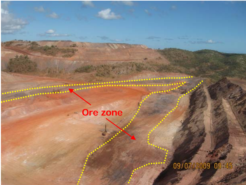
Figure 5 - Mullet Pit at the end of June 2009 looking west with the development of the permanent haul road into the Mullet Acacia ore zones
