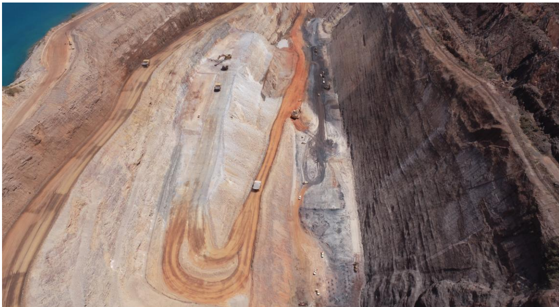
Figure 2: Koolan Island Main pit, eastern half, showing excavation of the former eastern mine haul ramp (underway at centre) and high grade ore mining along the footwall (right hand side), September 2024.
