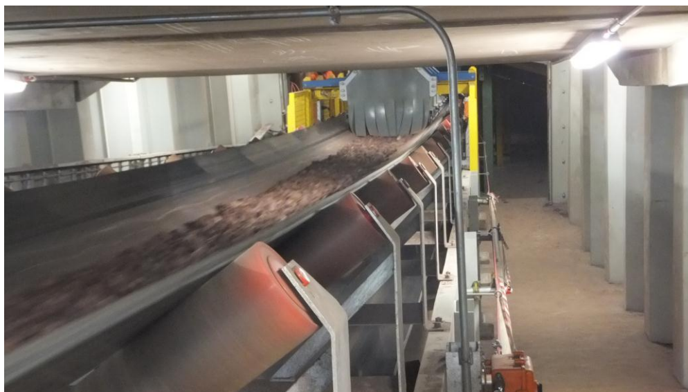
Figure 4– The new unloader in action.
